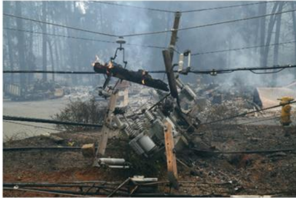
Power lines near Paradise, Calif., during the Camp Fire, which was ignited last year by Pacific Gas & Electric equipment. Jim Wilson/The New York Times
